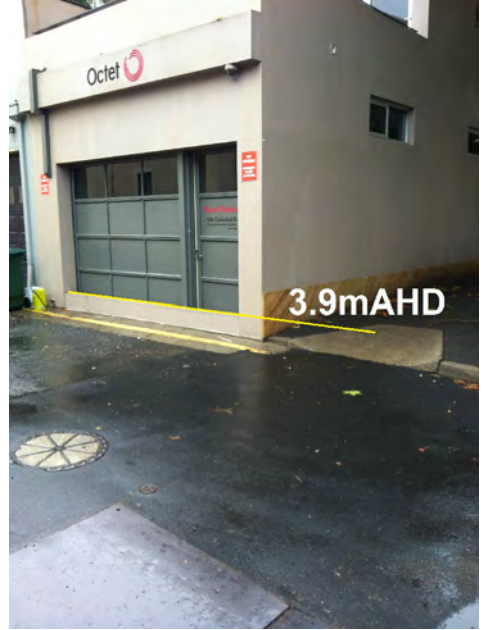
Flood barrier installed at Bossley Terrace, with approximate elevation of barrier height.
